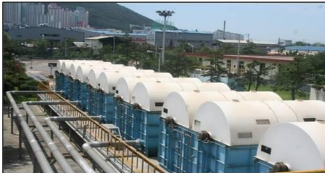
Smart Units, Tongbok Wastewater Treatment Plant, South Korea
